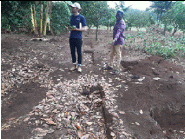
Drainage tunnels for preventing soil erosion
