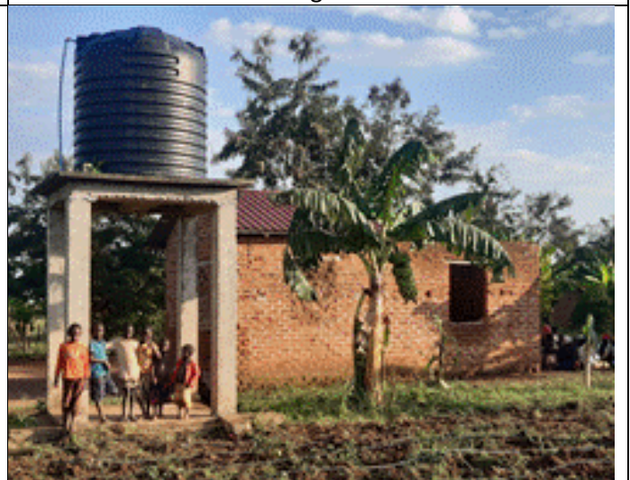
Water storage for agricultural site (5 m 3 )
